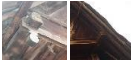
Figure 22. (a) Hooked notched corner joint with a peg at the bottom (b) Hooked corner notched joint
